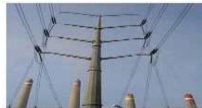
2. Tubular Steel Pole
