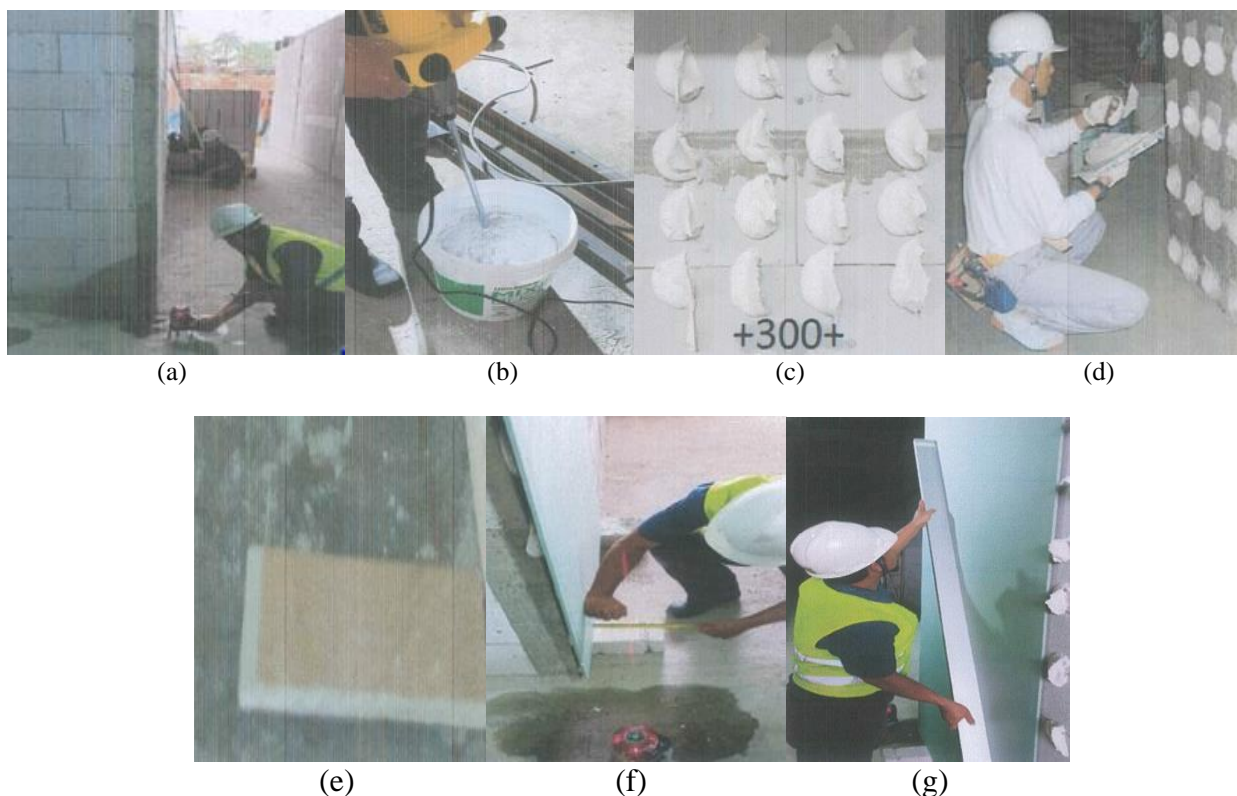
Figure 1. The stick on wall method: (a). Ensure verticality, (b). Mix the GL bond with water, (c). Start gluing, (d) Installing GL bond, (e) Gypsum supports on the floor, (f) Installing stick on wall, (g) Make sure the stick on wall flat. (Source: PT Total Bangun Persada)
