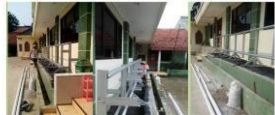
Fig. 8. Stage 3: Making Construction with Canal C Steel and Finishing of Fish Pond (Source: Team's Documentation, 2017)
